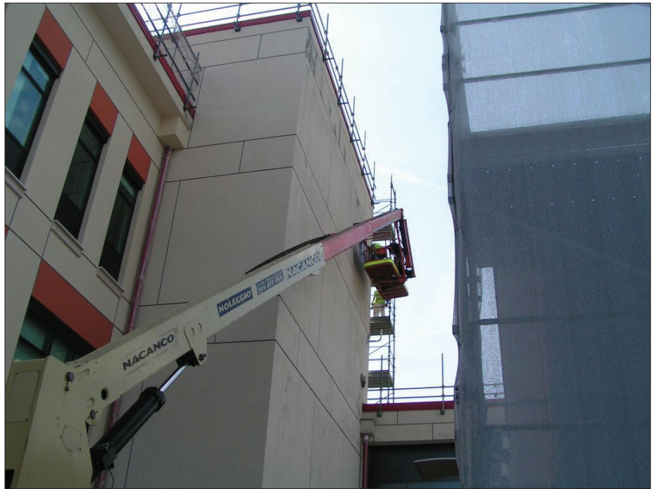
European construction often requires a host nation safety manager, in addition to any U.S. requirements administered by the Occupational Safety & Health Administration. PHOTO COURTESY MICHAEL-BRUNO LLC
